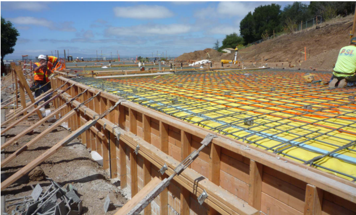
THE EARLY STAGES OF CONSTRUCTION FOR A NET ZERO, LOW-CARBON, LEED PLATINUM SCHOOL PROJECT, DESIGNED BY SIEGEL & STRAIN ARCHITECTS.
